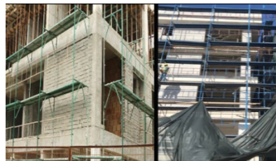
Figure 6. Better form of scaffolding system compared to Lebanon case
