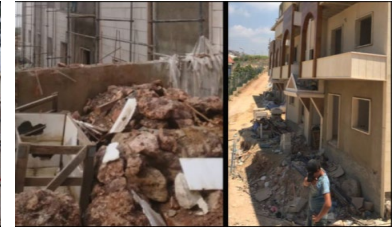
Figure 4. Messy surroundings and improper waste disposal
