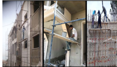
Figure 3. Disastrous form of scaffolding and absence of PPE
