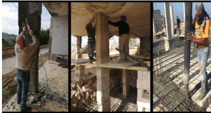
Figure 2. Workers undergoing construction activities without PPE
