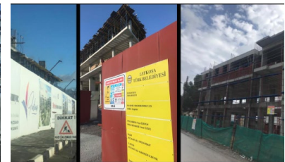
Figure 7. Presence of warning signs and barriers
