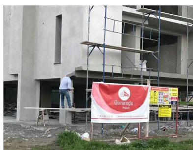
Figure 10. A worker performing plastering without any PPE in a small construction company
